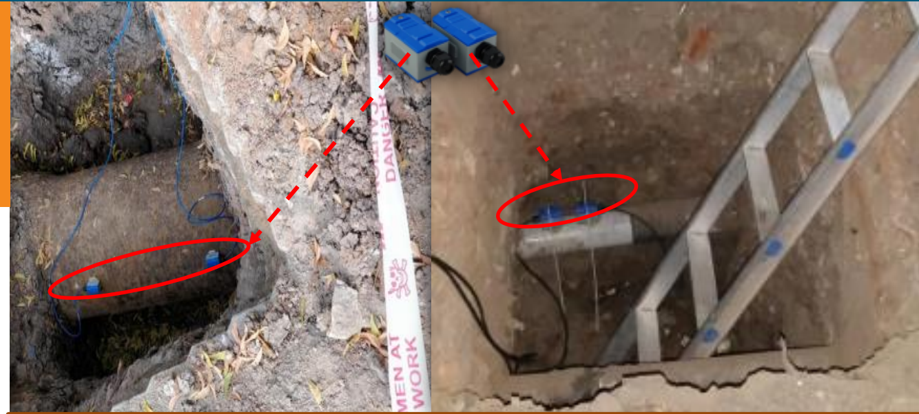
Flow & Pressure measurement @ RS Puram, Coimbatore
