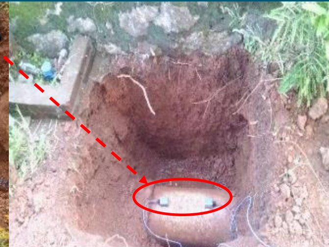
Flow measurement @ OHT common outlet
