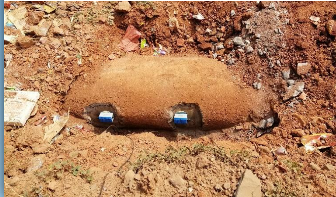
550mm, Transmission Line Concrete Lined Mild Steel Pipe
