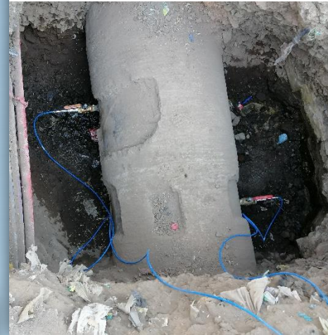
700mm, Transmission Line Concrete Lined Mild Steel Pipe
