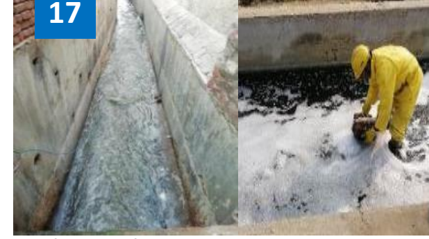
Verification Of Existing Meter At STP Inlet: ❑ Observed more than 15% measurement error.
