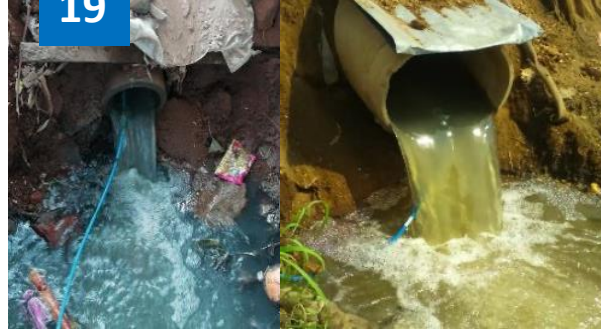
Municipal Corporation 2 - Sewage Flow Quantification For New STP Design: ❑ Recorded particularly higher flow values around midnight.
