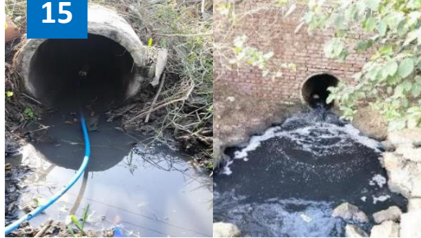
City 1 - Open Sewage Discharge Into River, Multiple Measurements Under A City-wide Wastewater Discharge Monitoring Scheme: ❑ For the purpose of river front development. ❑ Wastewater generated was 35% to 40% higher than the expected value.
