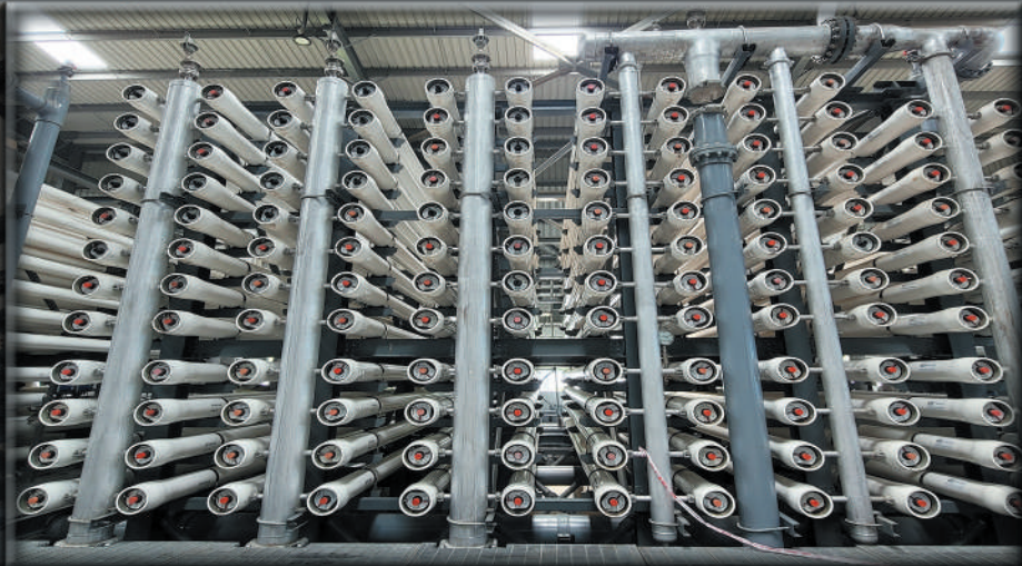
Plant Inlet Permeate and Drain Measurement
